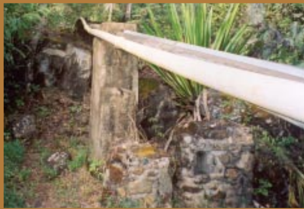
Gravity pipe at Mulanje, Malawi: the new pipe is strapped to the side of the original.
